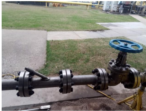
Figure C.6 Loop with Pneumatic Valve Uninstalled
